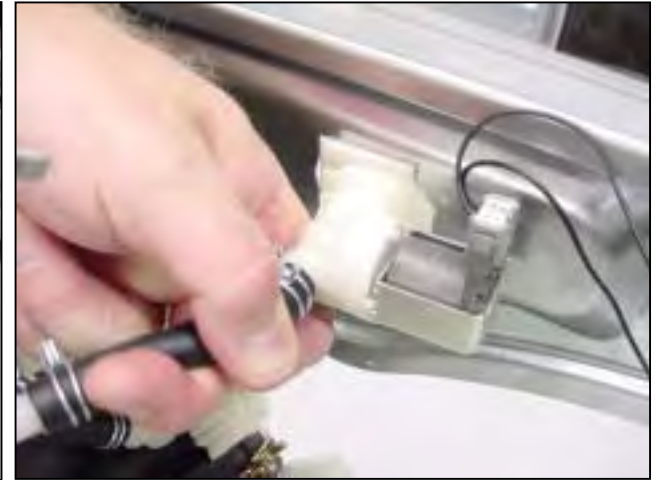
Disconnect hot water valve hose
