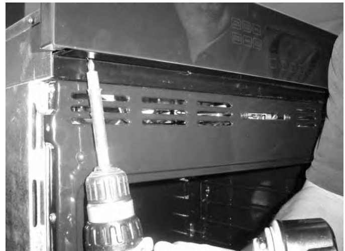
Screws on Bottom of Control Panel
