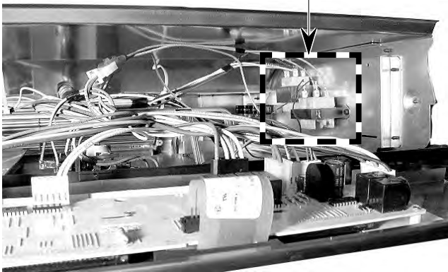
Oven Light & Control Power Transformers
