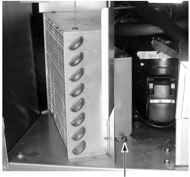
Condenser Fan Motor Bracket Bolts (1 of 2)
